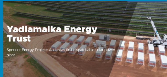
Invinity currently building Australia's first dispatchable solar power plant with an 8 MWh VFB coupled with a 6MWp solar array in South Australia
