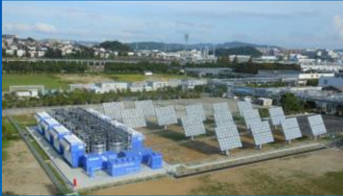
1 MW/5 MWh, Sumitomo - Japan
